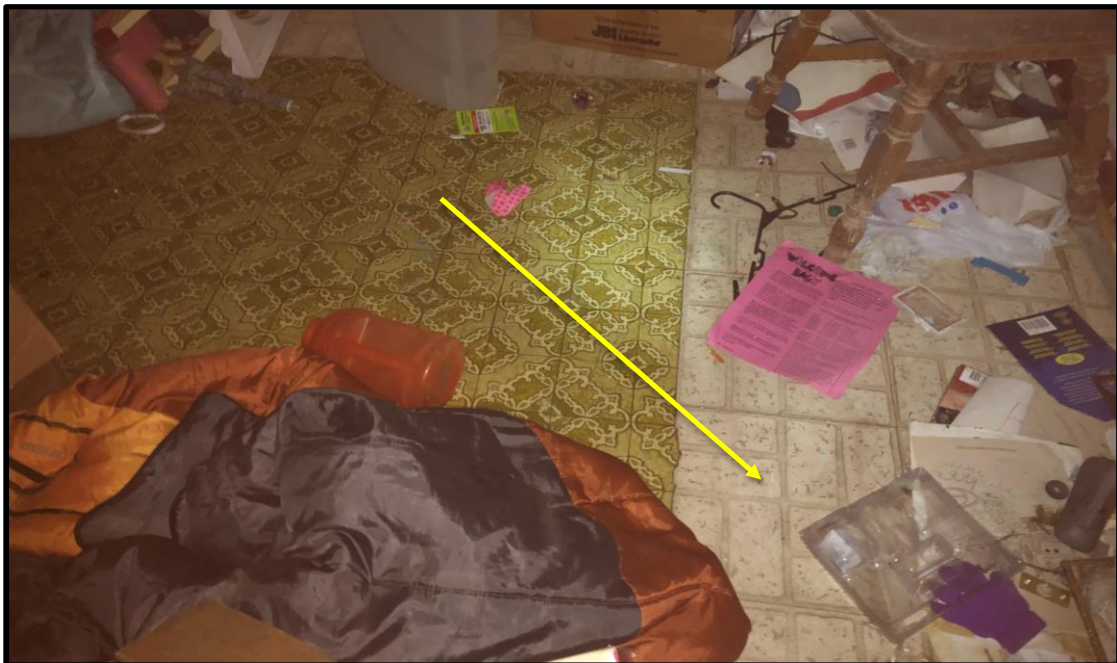
PHOTO: 2 DATE: 6/12/2019 BY: Greg Ross SUBJECT: HA 18: Asbestos-containing white floor tile in the first floor bedroom.
