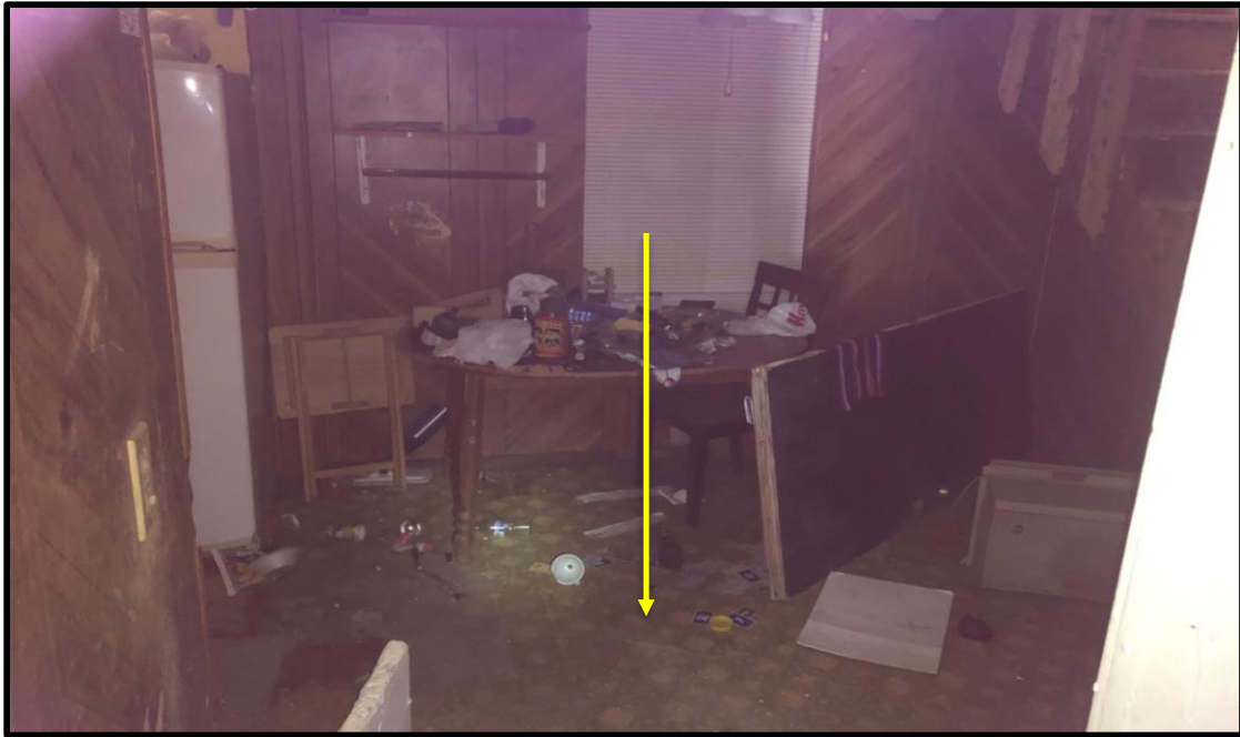
PHOTO: 1 DATE: 6/12/2019 BY: Greg Ross SUBJECT: HA 2: Asbestos-containing green flooring (with white square pattern) in the 1st floor hallway and dining room.
