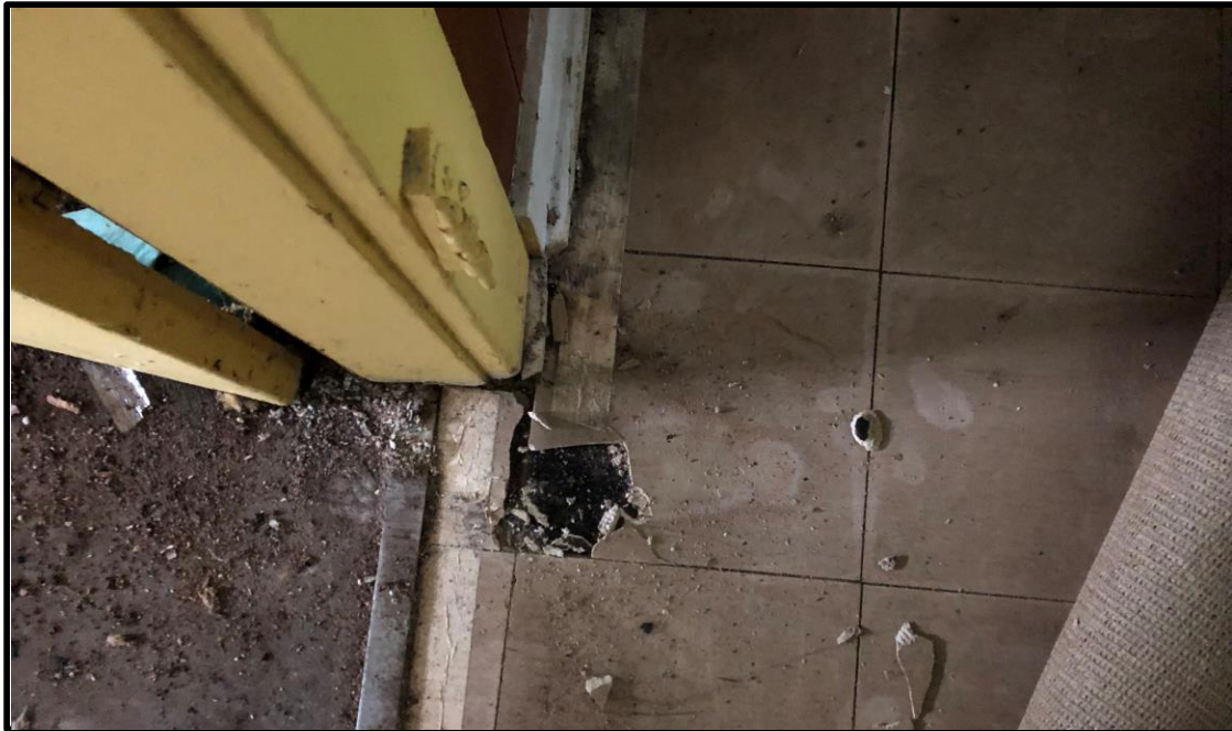
PHOTO: 1 DATE: 6/13/2019 BY: Greg Ross SUBJECT: HA 5: Asbestos-containing 9x9-inch tan floor tile and underlying mastic, under carpeting by back door.
