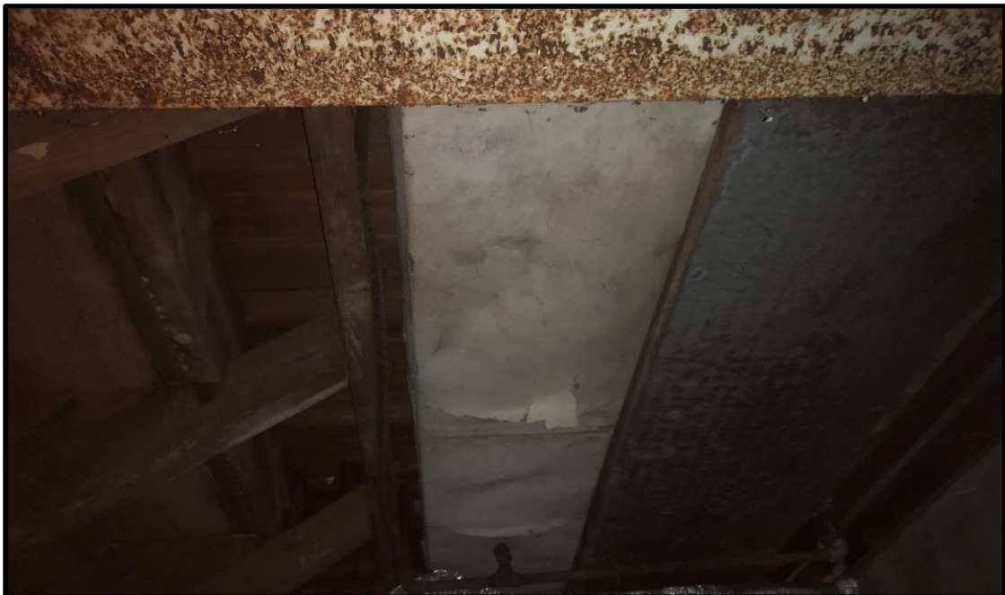
PHOTO: 2 DATE: 6/12/2019 BY: Greg Ross SUBJECT: HA 9: Presumed asbestos-containing duct wrap on a basement ventilation run.
