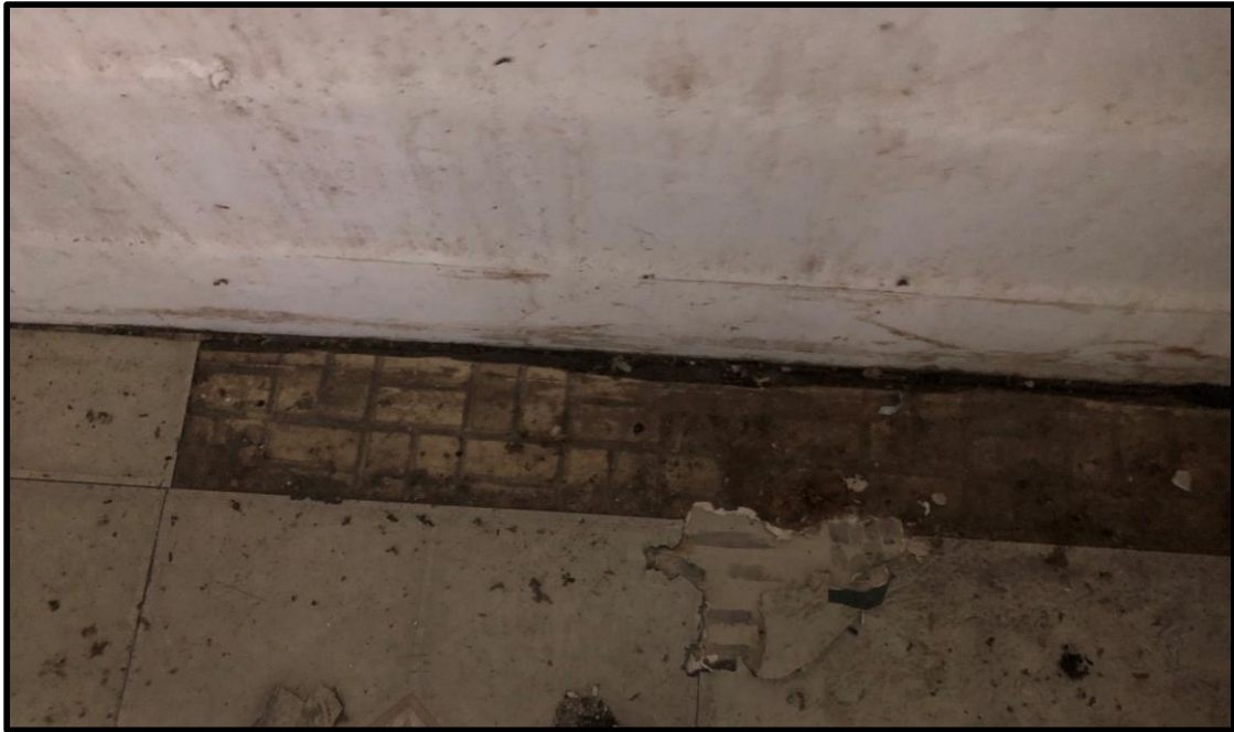
PHOTO: 1 DATE: 6/12/2019 BY: Greg Ross SUBJECT: HA 3: Asbestos-containing yellow/tan laminate flooring with a rectangle pattern - 1st floor bathroom under HA 2.
